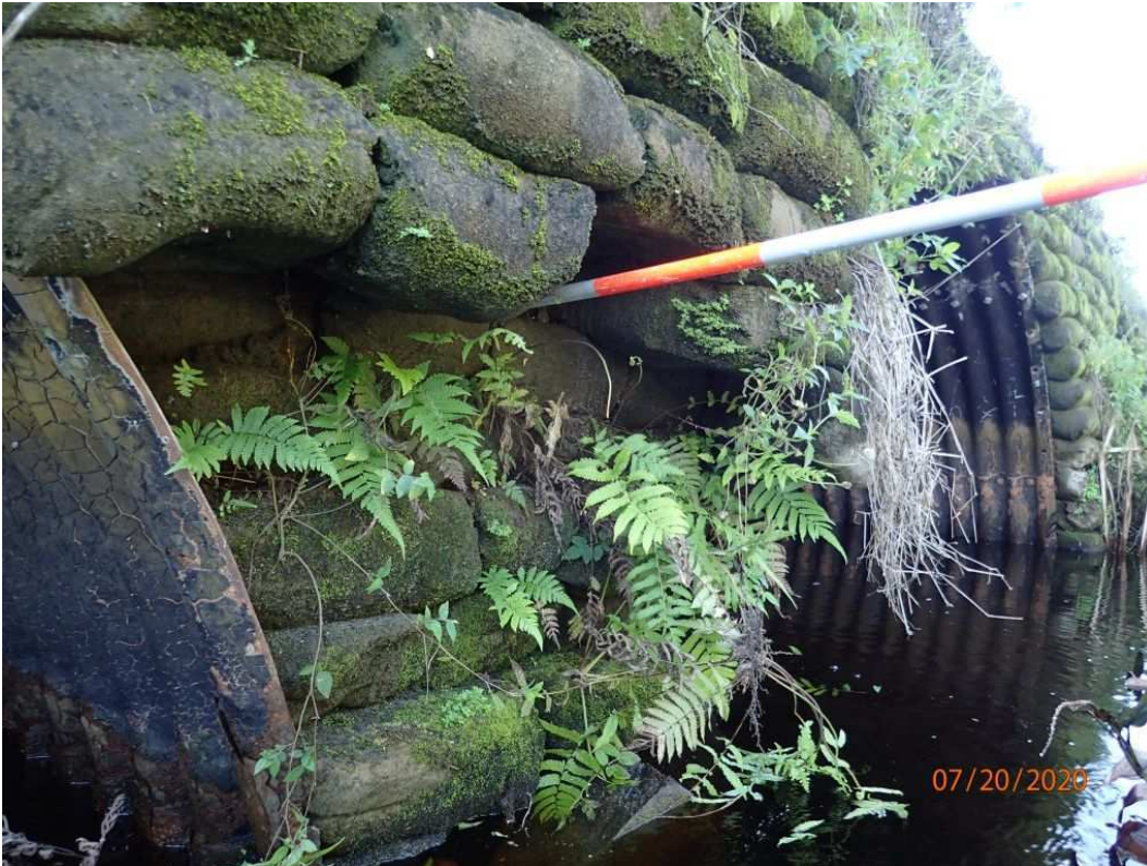
Photo 5: Element 8477: Vegetation growing through the joints of the west headwall
