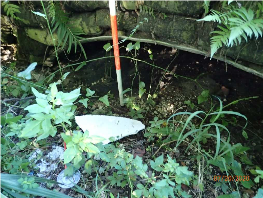
Photo 1: Element 8290: Build up in Pipe 1
