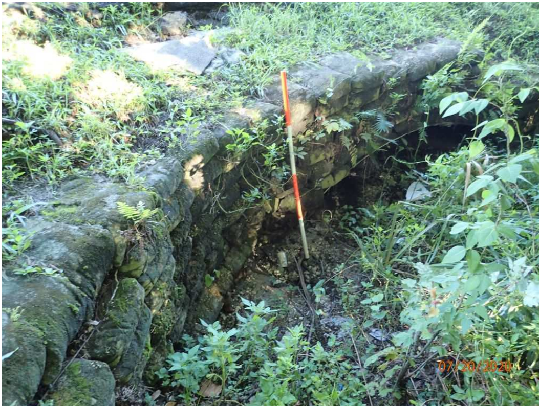
Photo 4: Element 8477: Settled sand cement rip rap bags in the east headwall over Pipe 1
