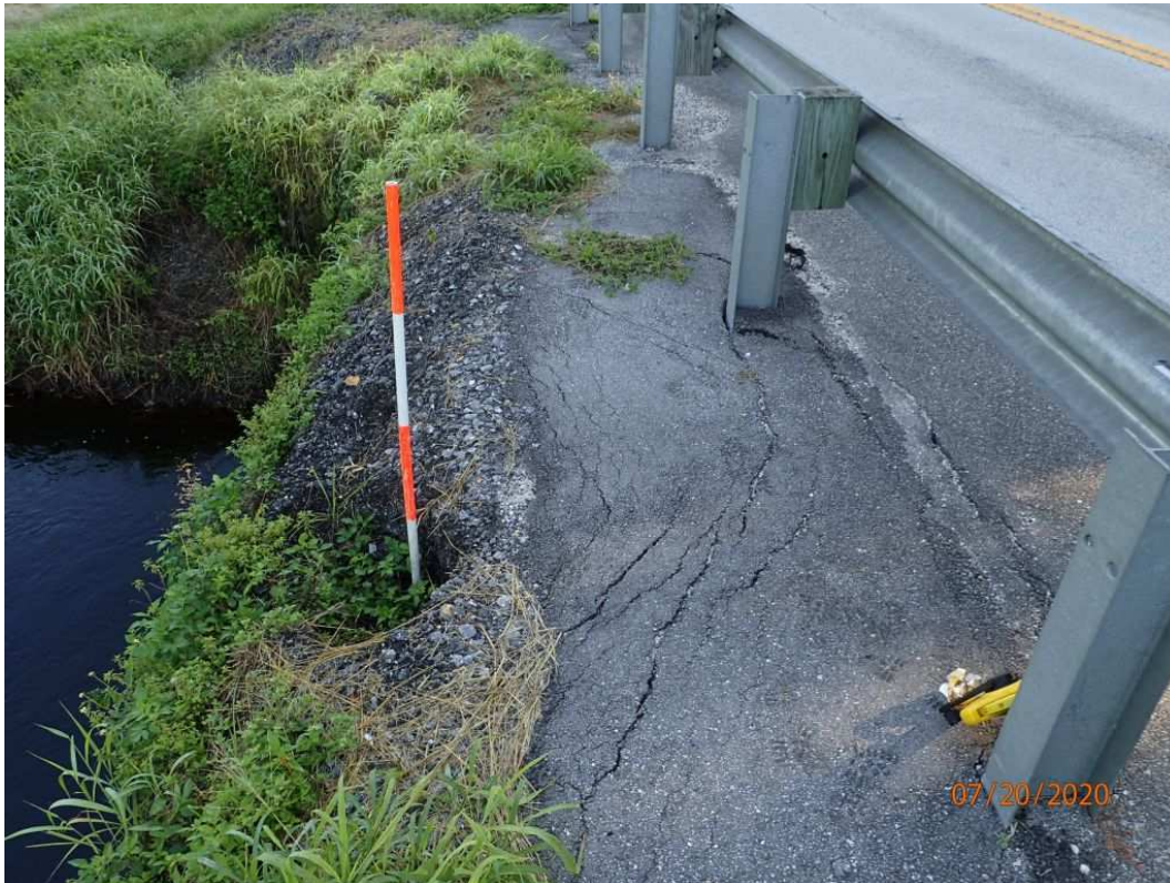
Photo 10: Inspection Notes: Depression over Wall 4 in the asphalt mowing strip
