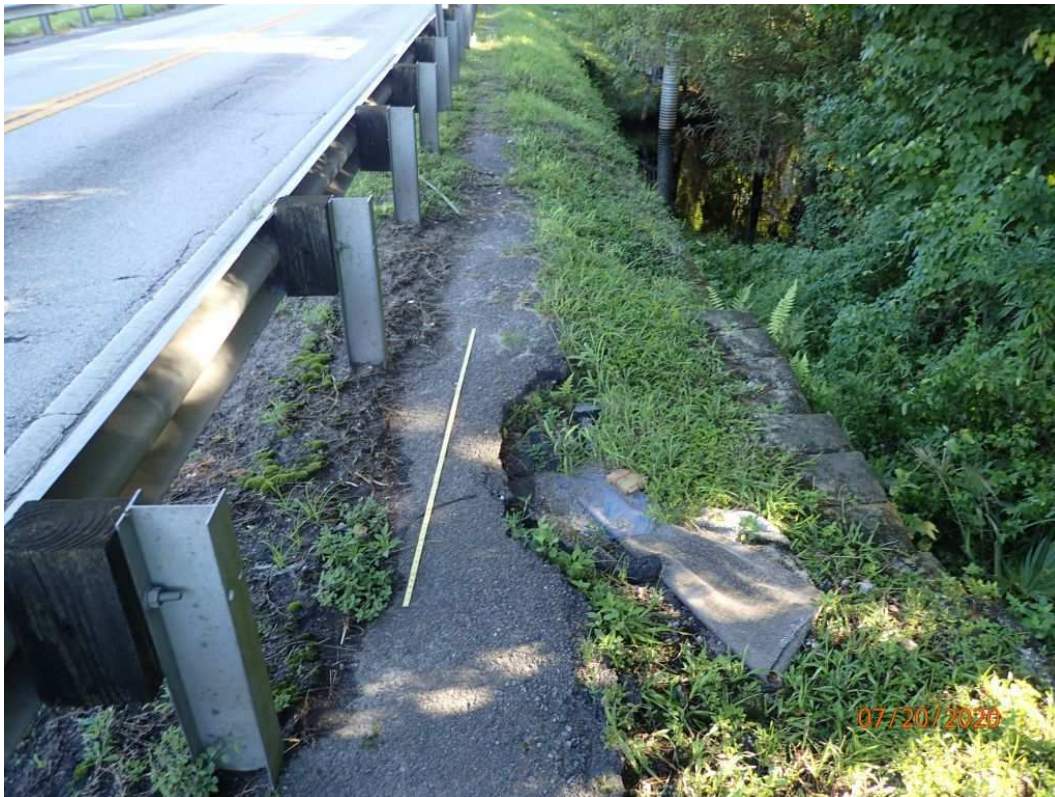
Photo 9: Inspection Notes: Washout in the west asphalt mowing strip
