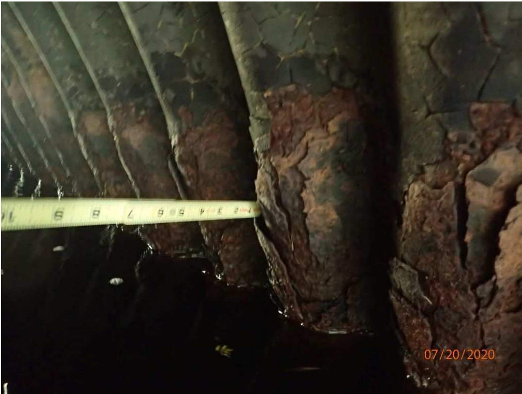
Photo 6: Element 240: Delaminative corrosion on pipes sidewalls and connecting hardware and failed bituminous/galvanized coatings of pipes
